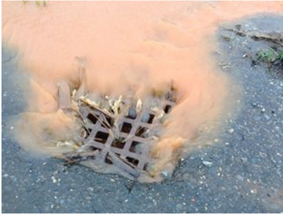
A stormwater inlet receiving polluted runoff. Photo courtesy of the City of Lynchburg
